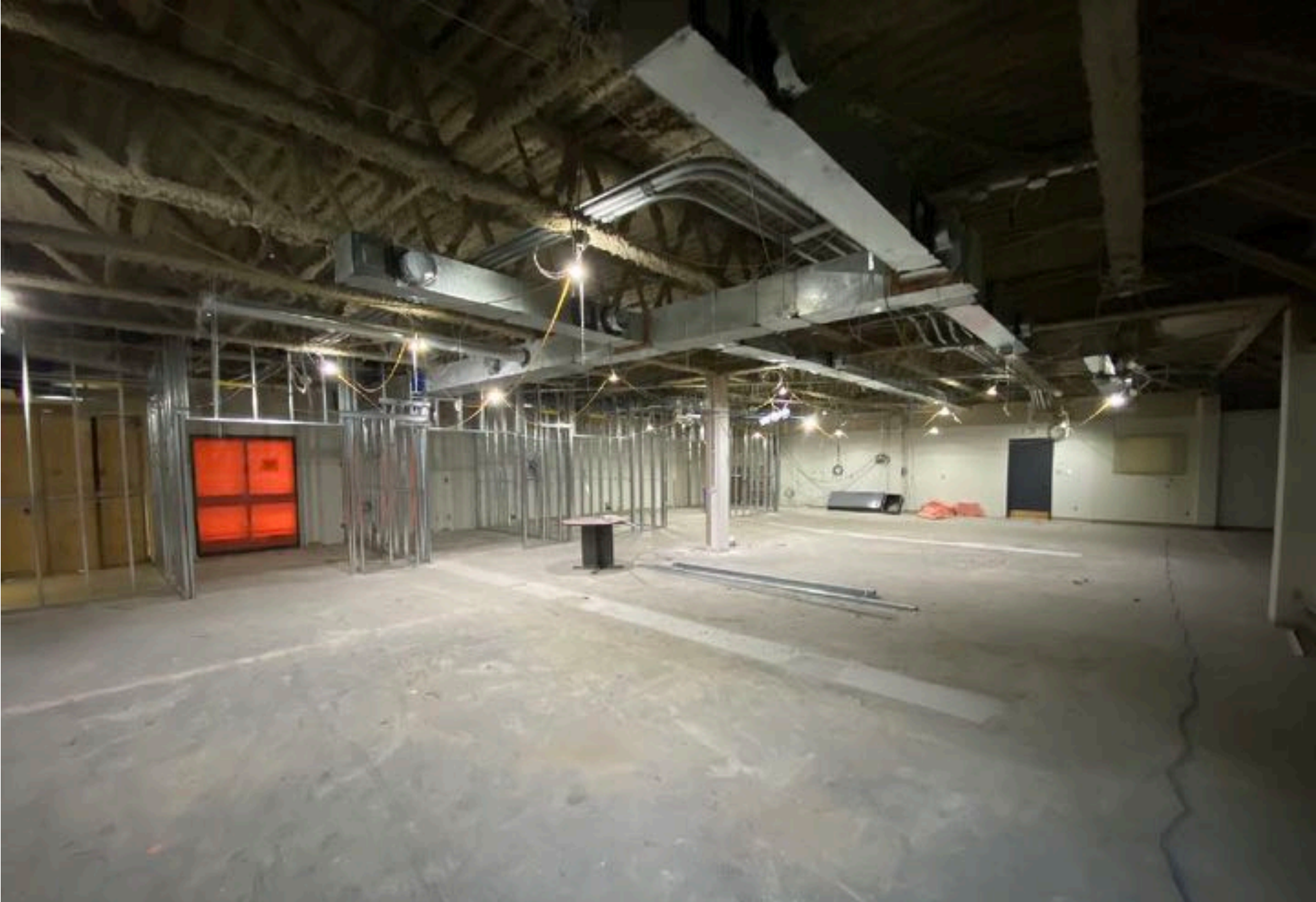
UTS Back of House Work Area
